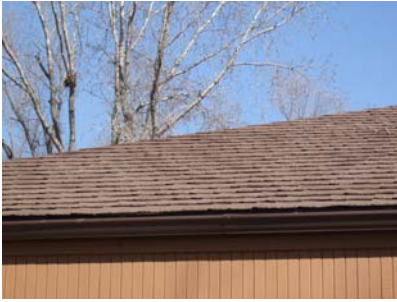
Roof where Rain Falls
